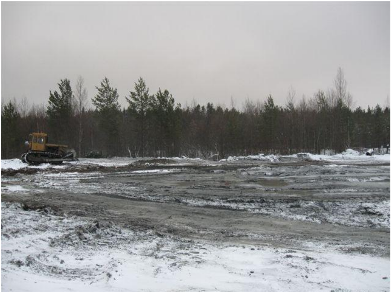
Figure 19. Overview of Oil Storage in Pokrovskoye, Onega Rayon (after completion of levelling operations)
